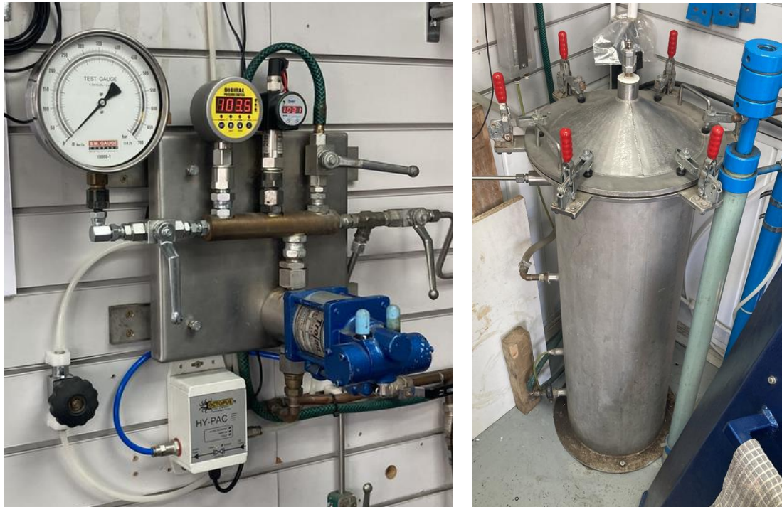
Figure 4: 7Z Hydro test system
