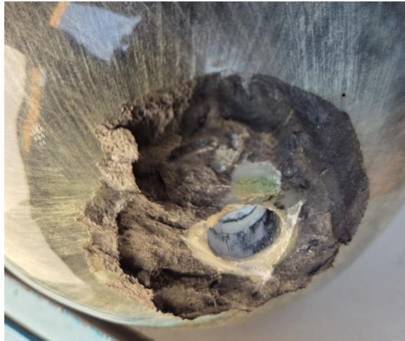
Damaged cylinder base
